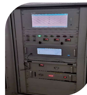
Online monitoring equipment
